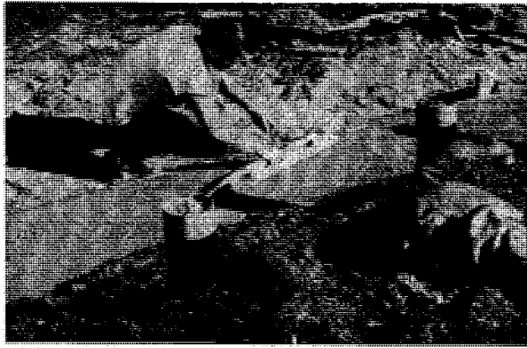
No project is complete until it is finished. Project Transition's Cement Masonry Course students learn this as well as other specific jobs during the 220 hours of classroom and field training they receive. (U.S.)
